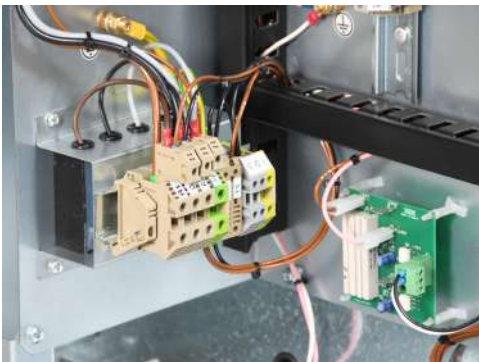
Fig 11 - incoming power terminals
